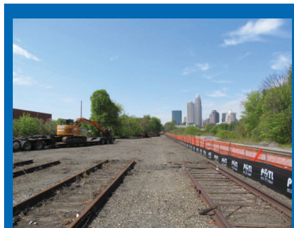
CATS will remove 5 of 7 sets of tracks on 16th Street providing you with a smoother drive in the future.
