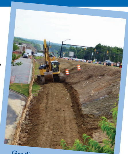
Grading starts for the largest wall along the alignment at the Mallard Pointe Shopping Center.
