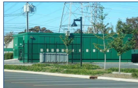
Typical LYNX Blue Line substation.
